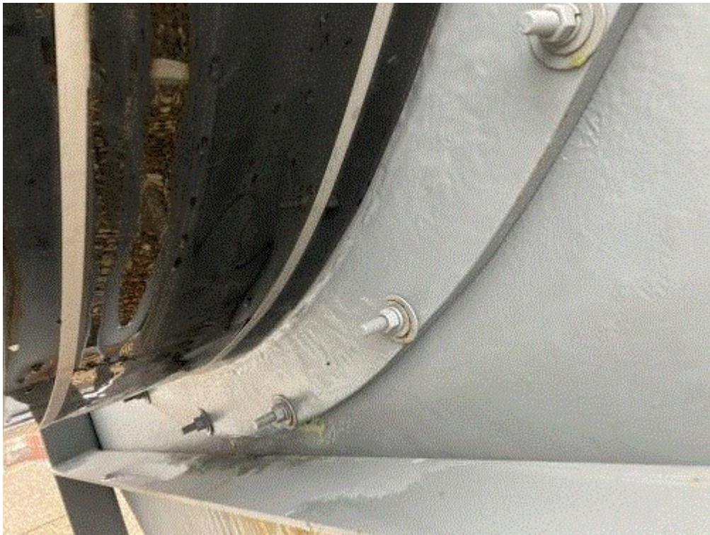
Image 2(EUCLINE) : Small drip of greenish liquid, bottom middle bolt area.
