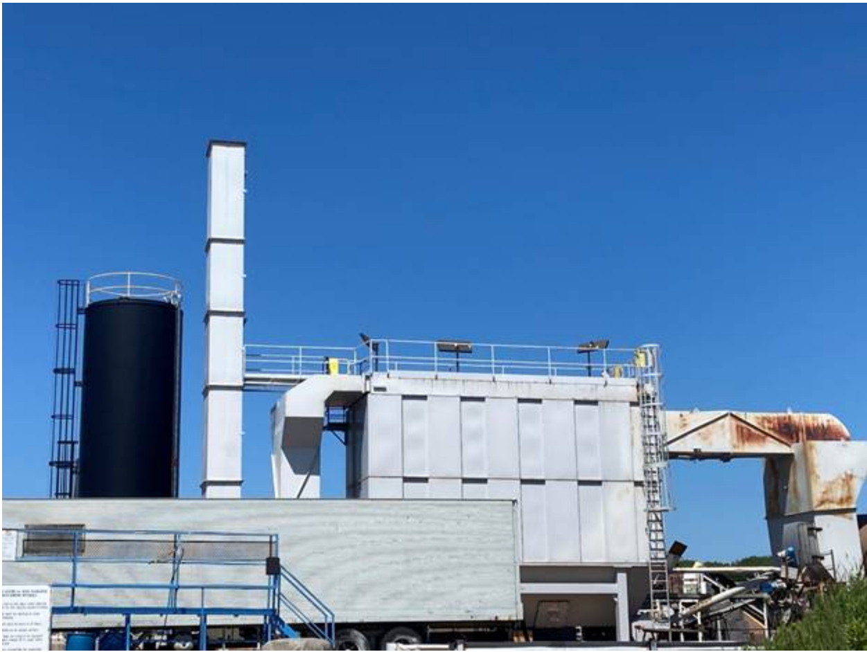
Image (2): Baghouse and stack
