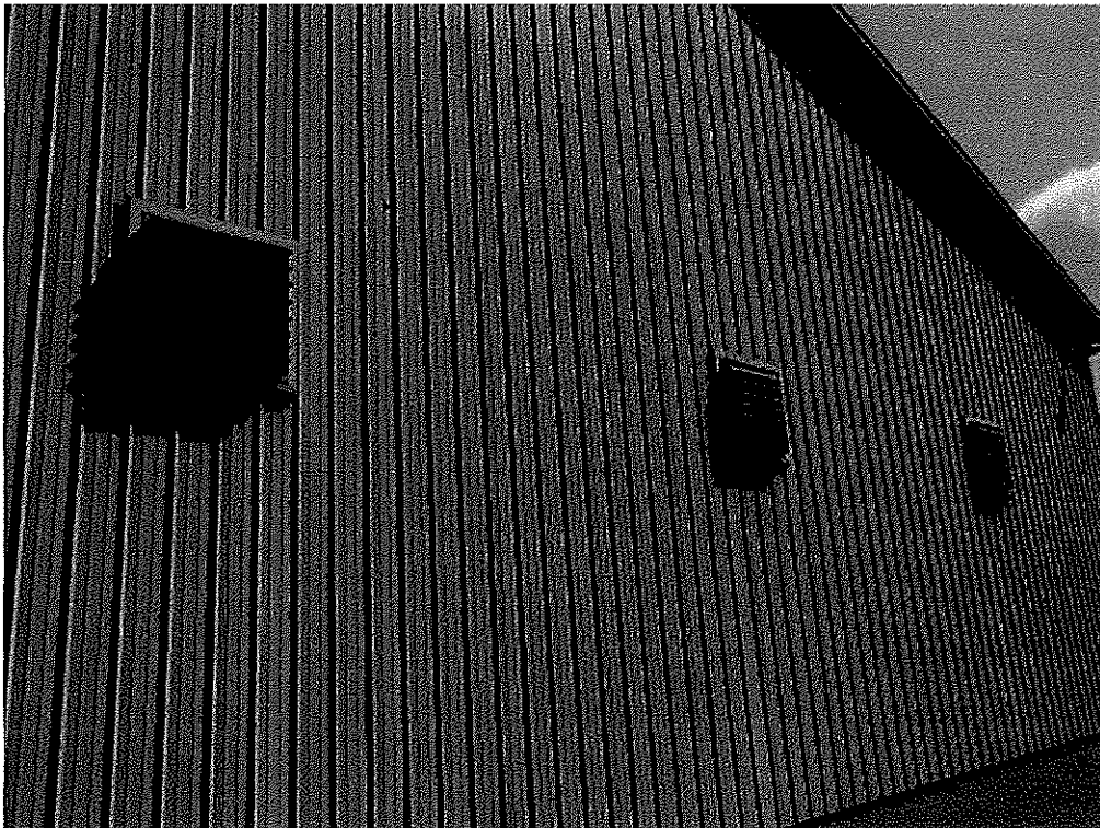
Image 6(4) : Exhaust vents from painting area
