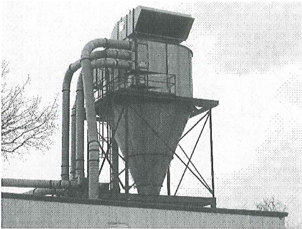
Image 2(Cyclone Photo 2) : This photo shows the ductwork feeding the cyclone. There is a screen covering the rectangle to prevent any large pieces from being exhausted.
