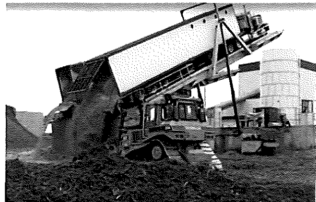
Figure 2-1. Wood biomass unloading
