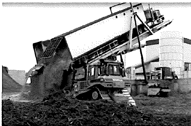
Figure 2-1. Wood Biomass Unloading
