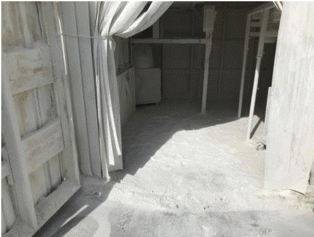
Image 3(Baghouse 3) : Interior of baghouse. Bottom of image shows where particulate escapes under door onto concrete pad outside.
