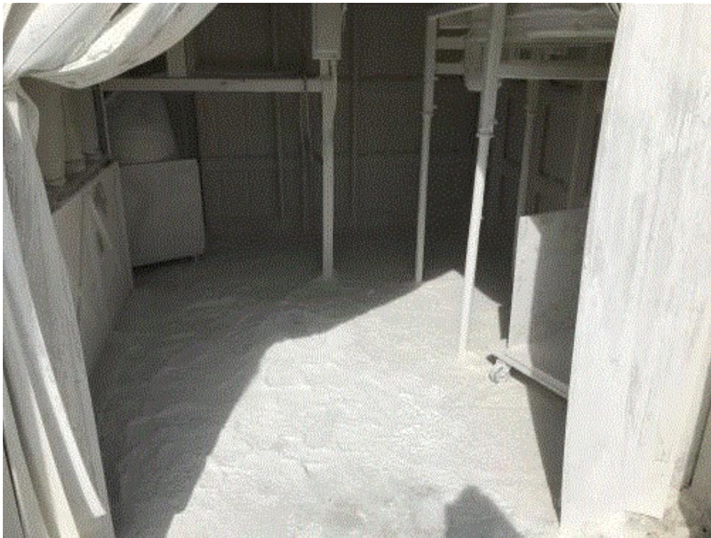
Image 2(Baghouse 2) : Interior view of baghouse.
