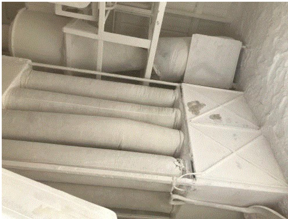
Image 1(Baghouse 1) : Interior view of baghouse.
