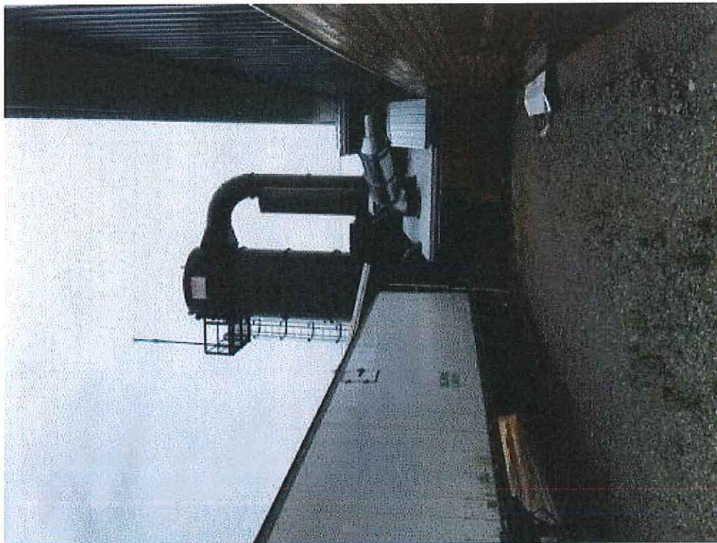
Image 1(Baghouse 1) : Baghouse for EUPNEUMATICLINE1.
