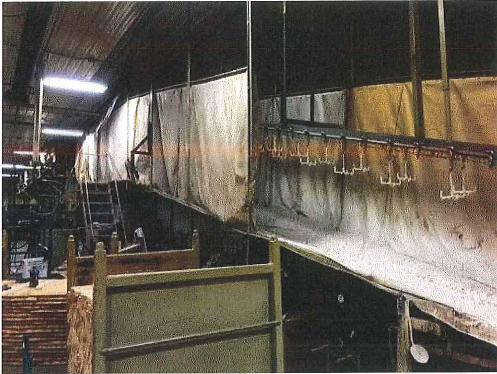
Image 4(Drying Carousel) : A drying carousel with fans blowing room temperature air. Emissions are exhausted to the general in-plant environment.
