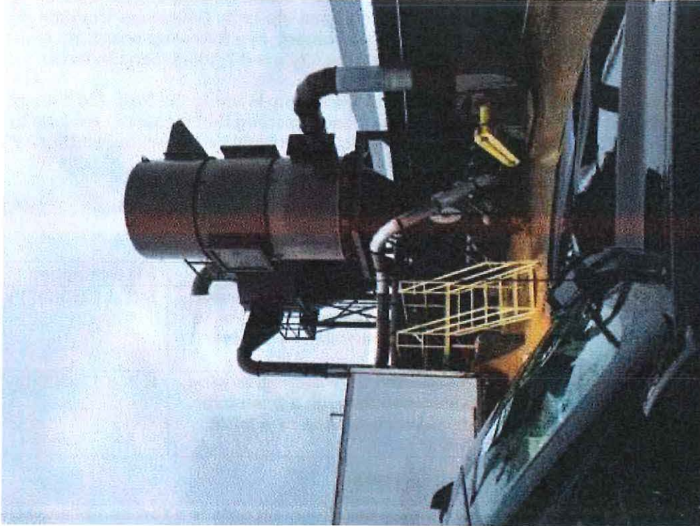
Image 2(Baghouse 2) : Baghouse for EUPNEUMATICLINE2.
