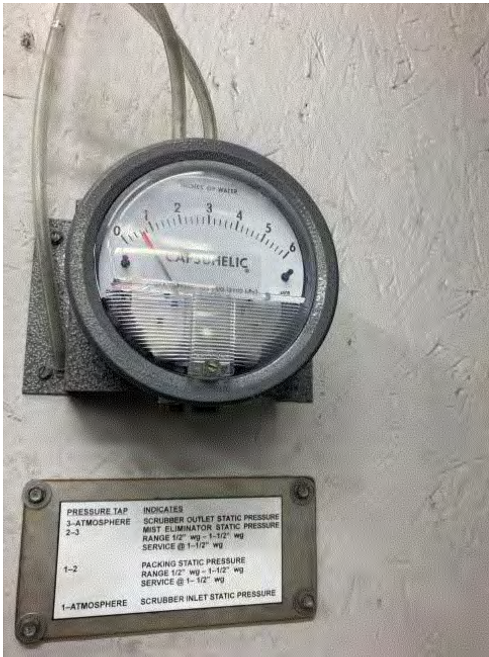
Image 2(Orthophos gauge) : Pressure drop gauge indicating the mist eliminator for the orthophosphoric acid tank is being operated properly.
