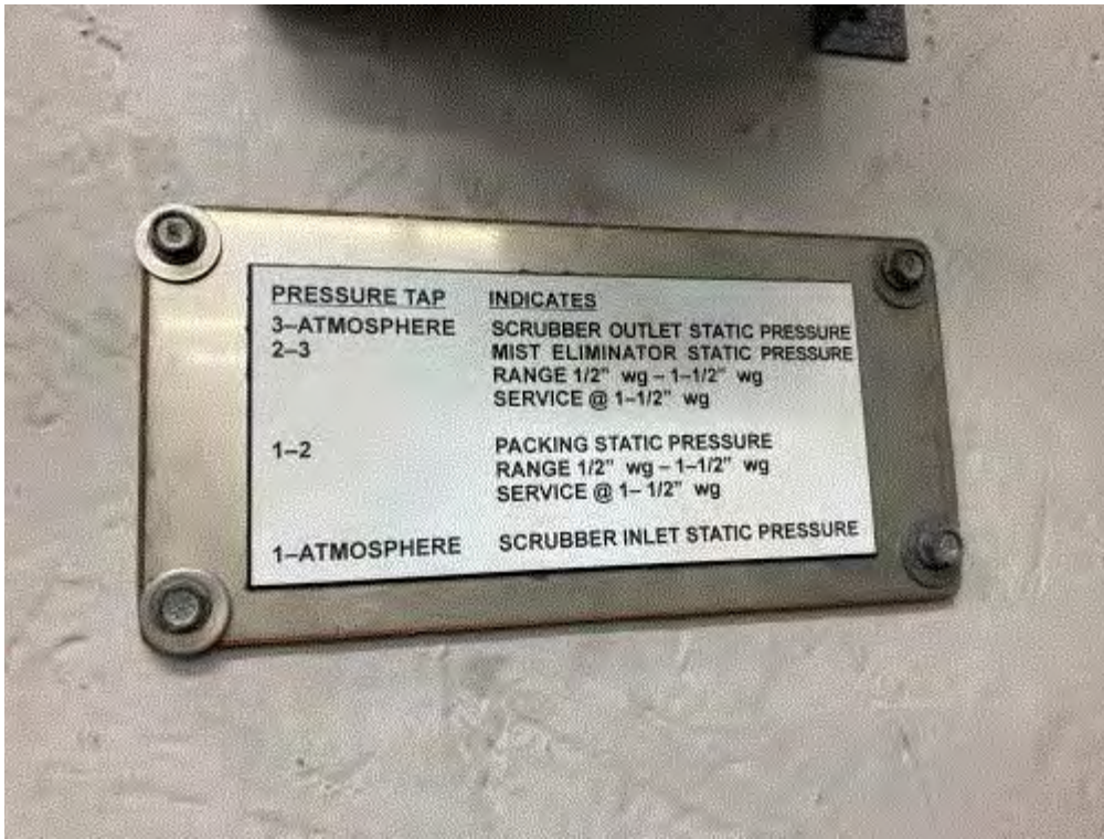
Image 1(Orthophosphoric #1) : Plate describing range within which proper operation occurs on the mist eliminator of the orthophosphoric acid tank exempt under Rule 291
