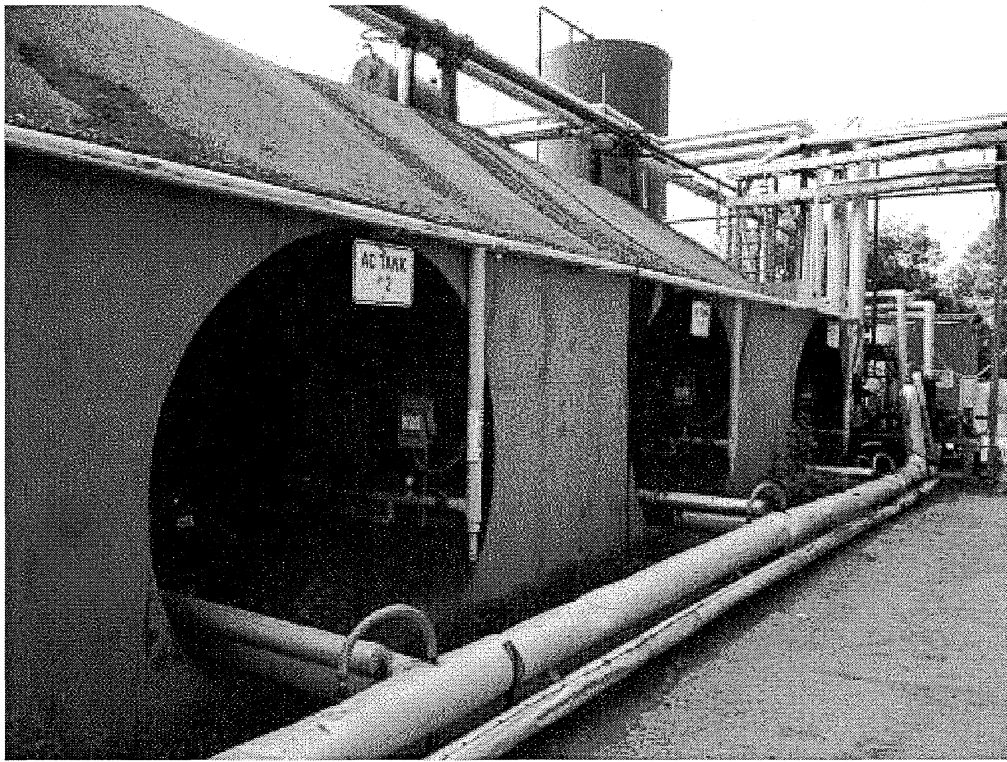
Image 13(Figure 13) : The liquid asphalt cement (LAC) storage tanks, 8/22/15, 10:42 am.
