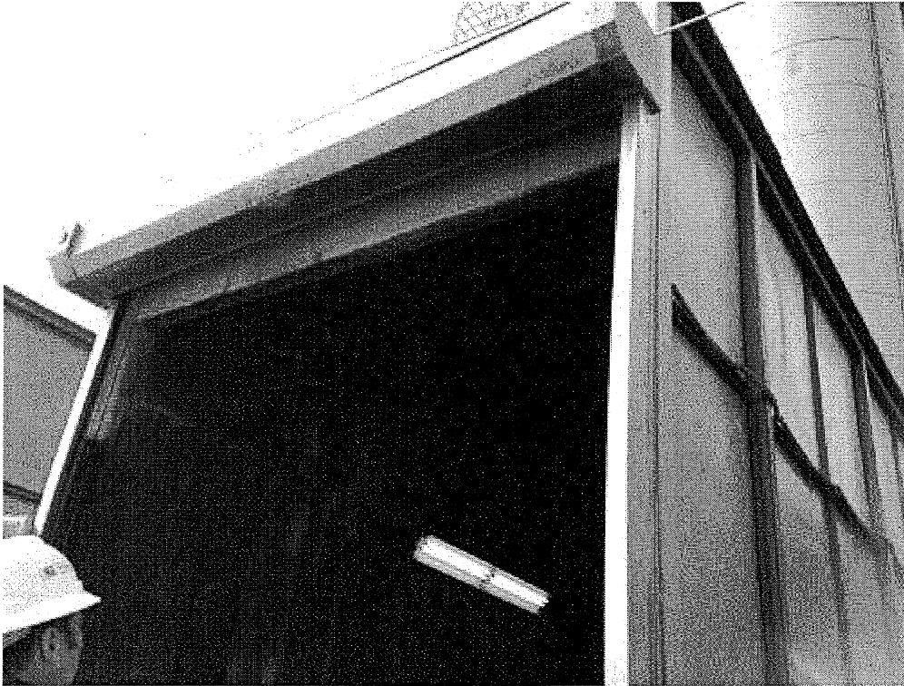
Image 8(Figure 8) : Missing curtain on the silo loadout enclosure entrance, 8/22/15, 10:36 am.
