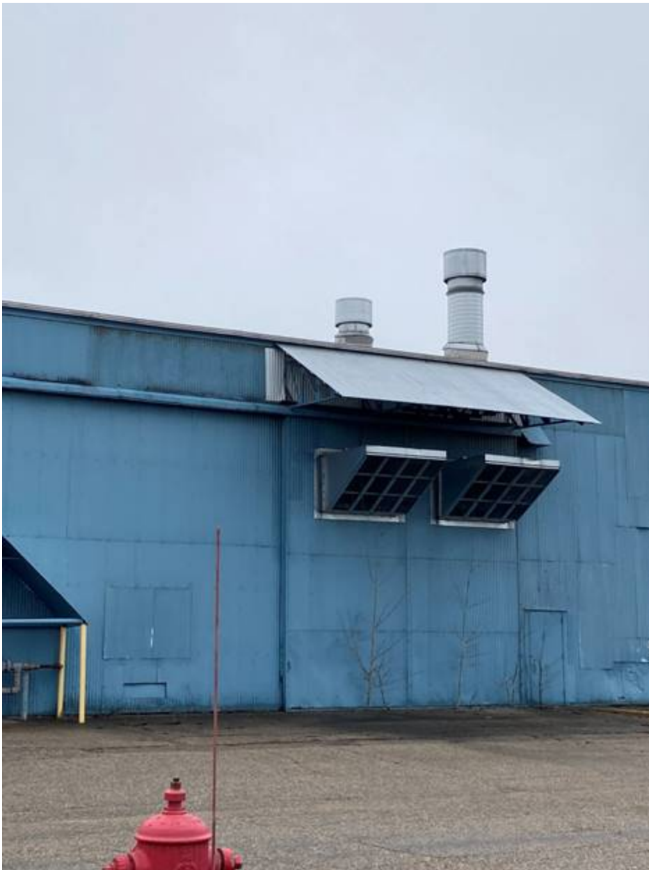
Image (2): PAINT SPRAY BOOTH INTAKE AND STACKS.
