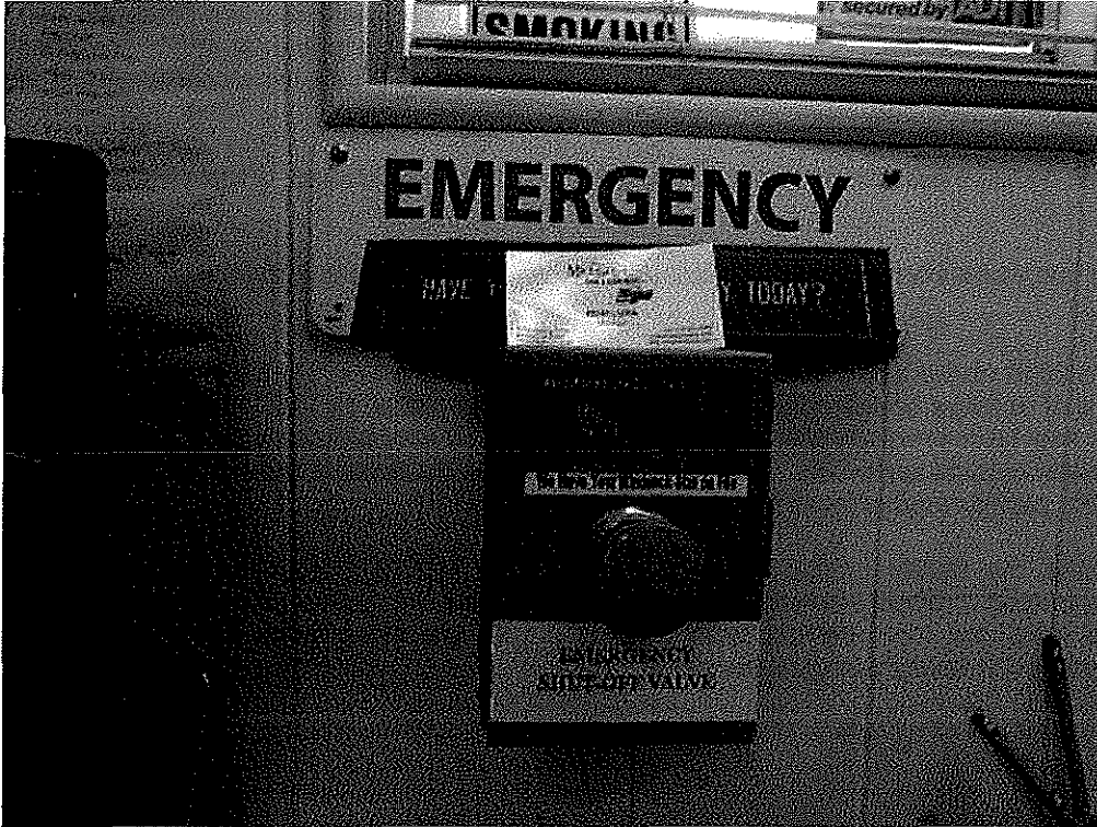
Image 1(1) : Shut-off valve in office
