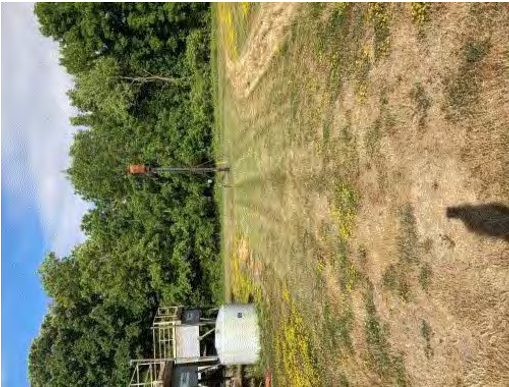
Image 1(900 scfm flare) : Disconnected "old" 900 scfm flare
