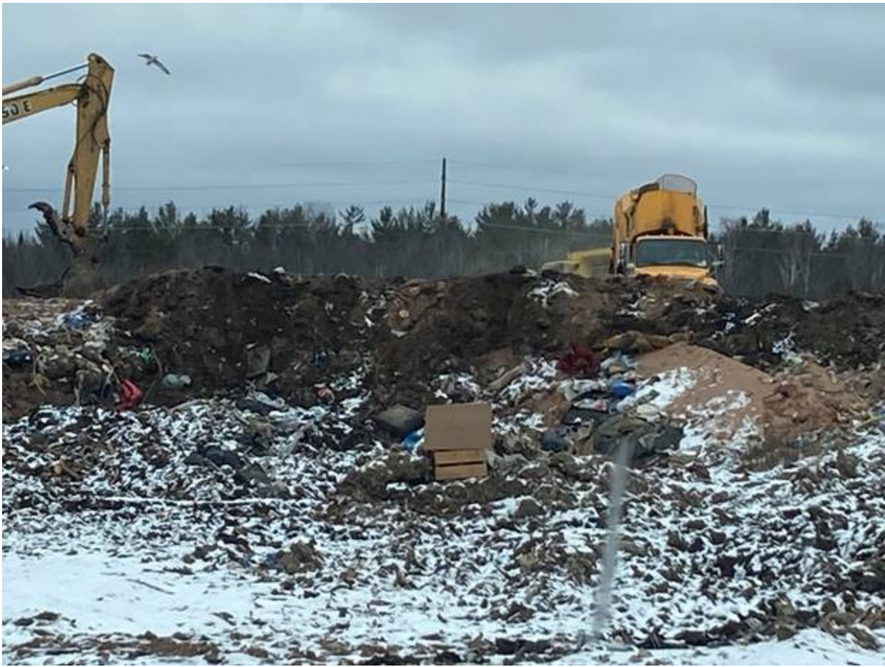
Image 3: Asbestos in cell 6 (uncovered)
