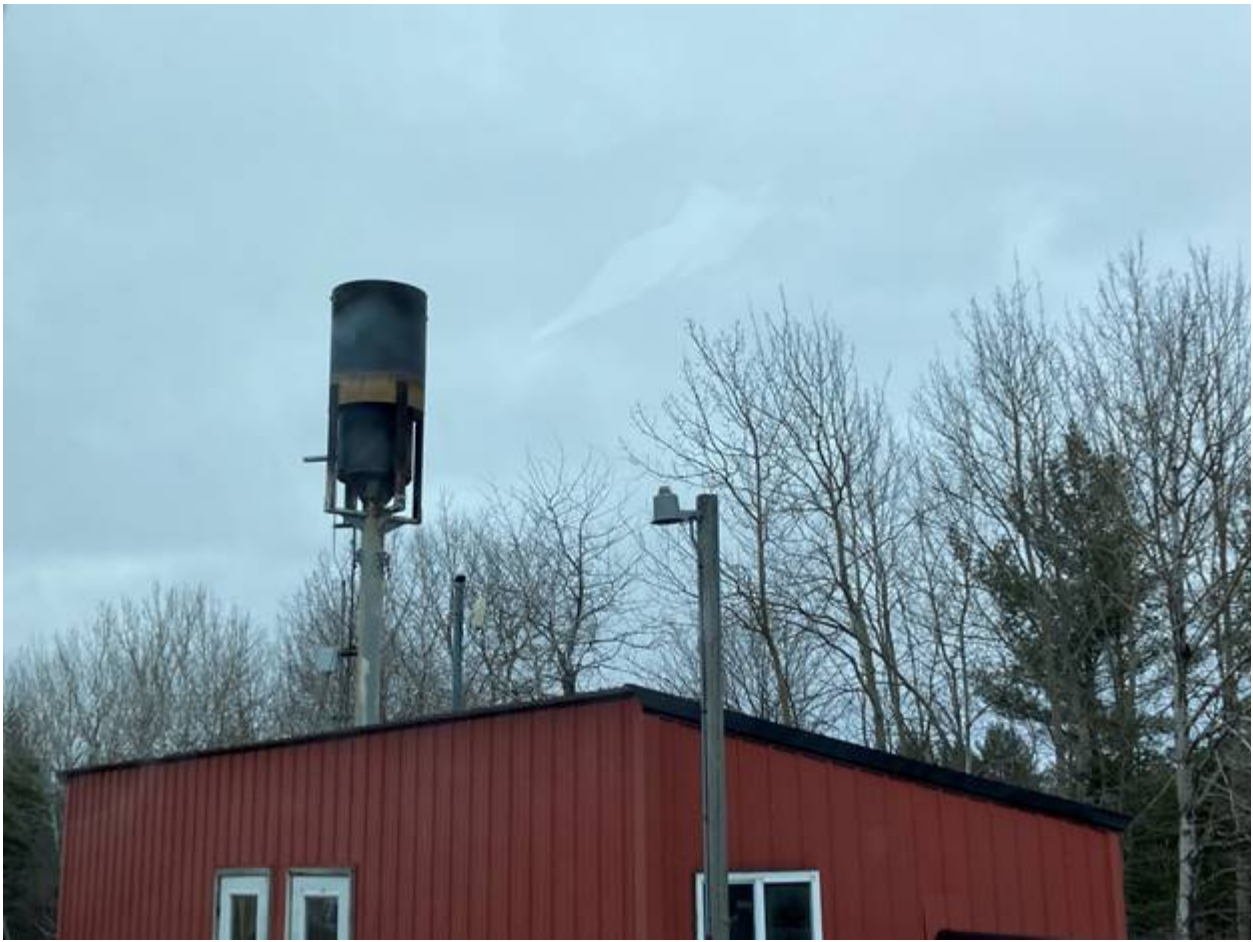
Image 1: South Landfill flare
