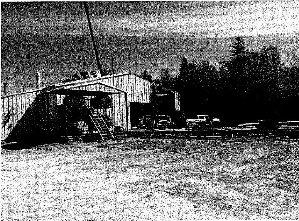
Image 2(view from SW) : another southerly view, in this one the removal of the eastern wall for removal of old engine, and installation of new unit is more visible.
