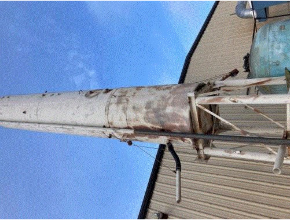
Image 2(EUSANDBLAST) : Sand storage tower.
