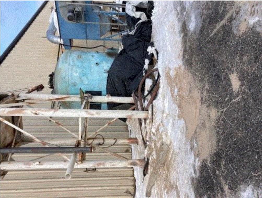
Image 3(EUSANDBLAST) : Base of sand storage tower and cartridge filter collector.
