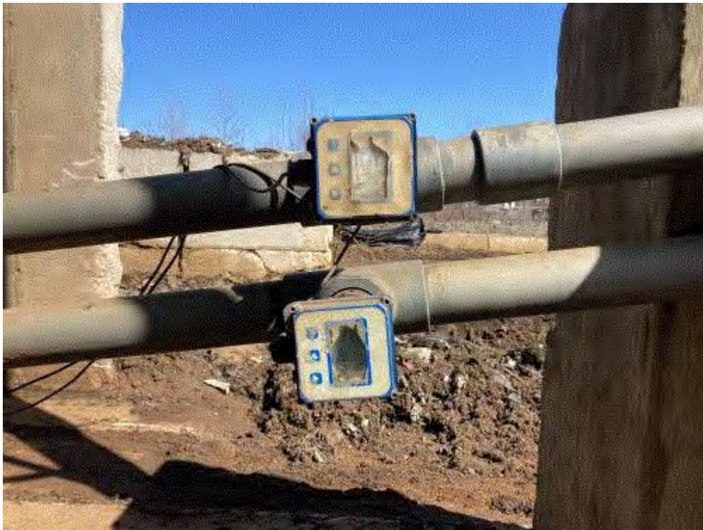
Image 3(3) : Broken water flow indicator and another broken gauge, the purpose of which was unknown.
