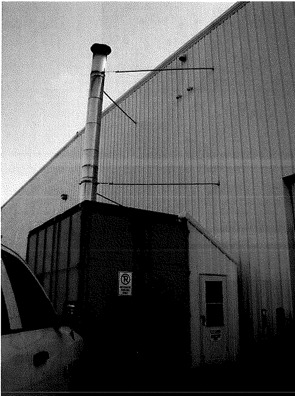
Image 7(Burnoff Oven) : burnoff oven stack - note the raincap
