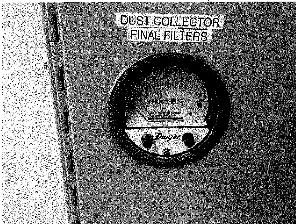
Image 5(Dwyer Pressure drop) : Photohelic pressure drop gauge used to monitor bag house pressure
