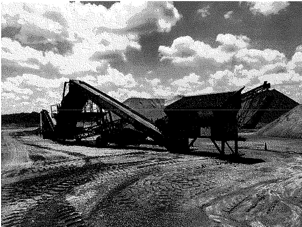
Image 5(030) : Dry screening plant
