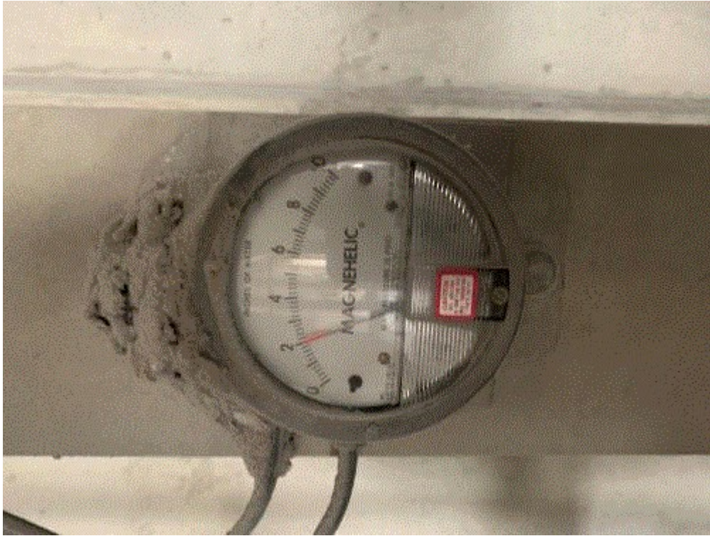
Image 6(Nu-Wool) : General baghouse room conditions (accumulation of material on gauges)
