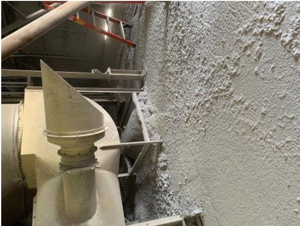
Image 1(Nu-Wool) : General baghouse room conditions (accumulation of material on the floor)
