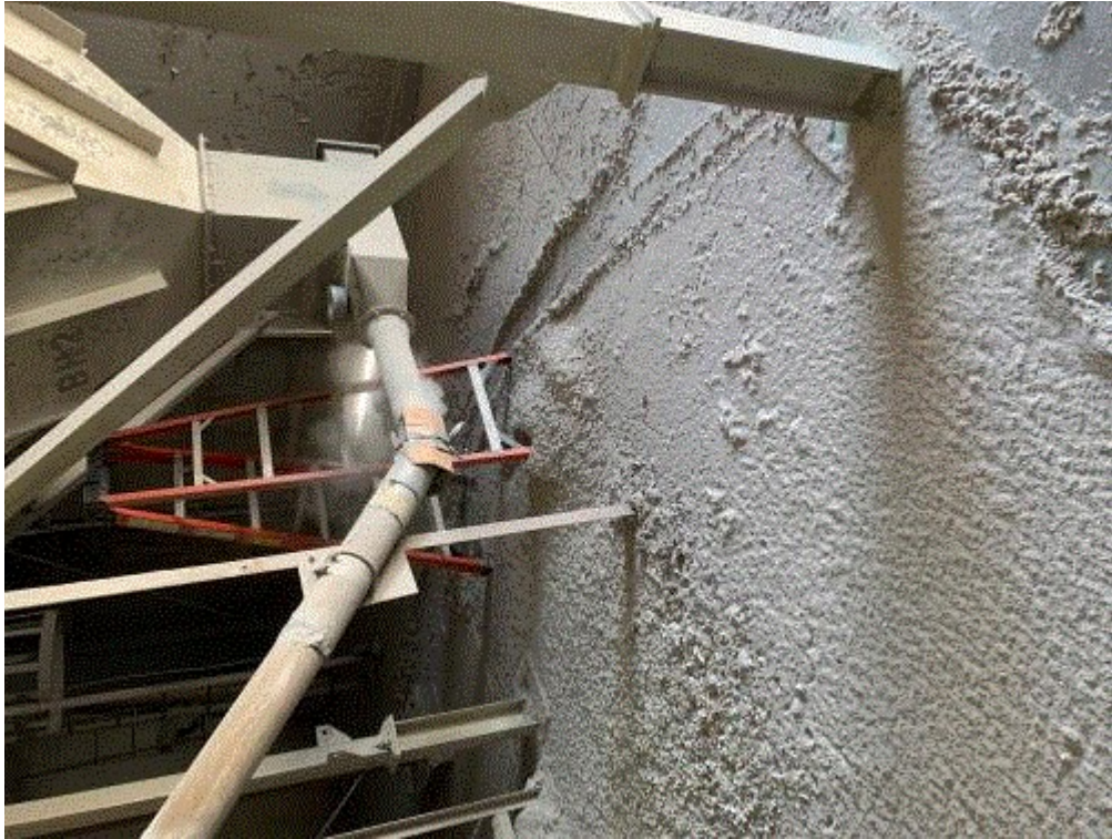
Image 4(Nu-Wool) : Leaking ductwork wrapped in cardboard
