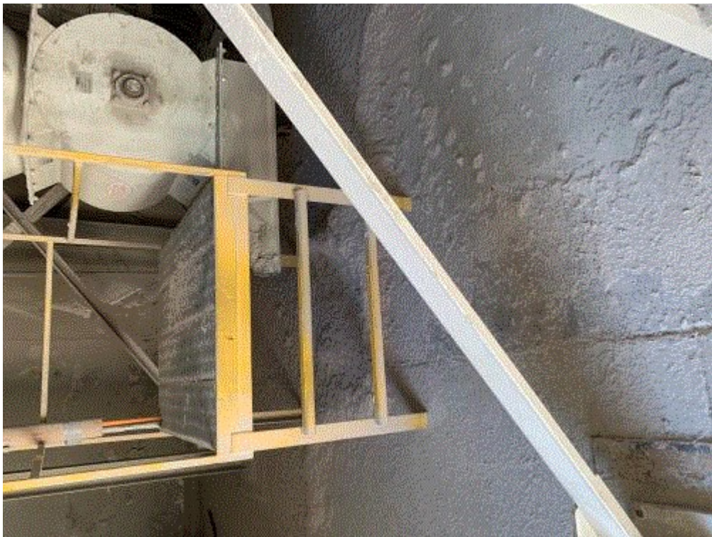
Image 5(Nu-Wool) : General baghouse room conditions (accumulation/piles of material under the baghouses)
