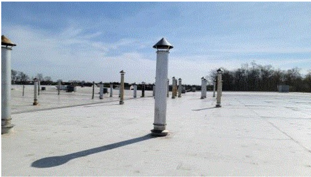
Image 5(Roof stacks) : Furnace roof stacks.
