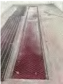
Image 2(Used filters) : Photo of filter prior to changeout
