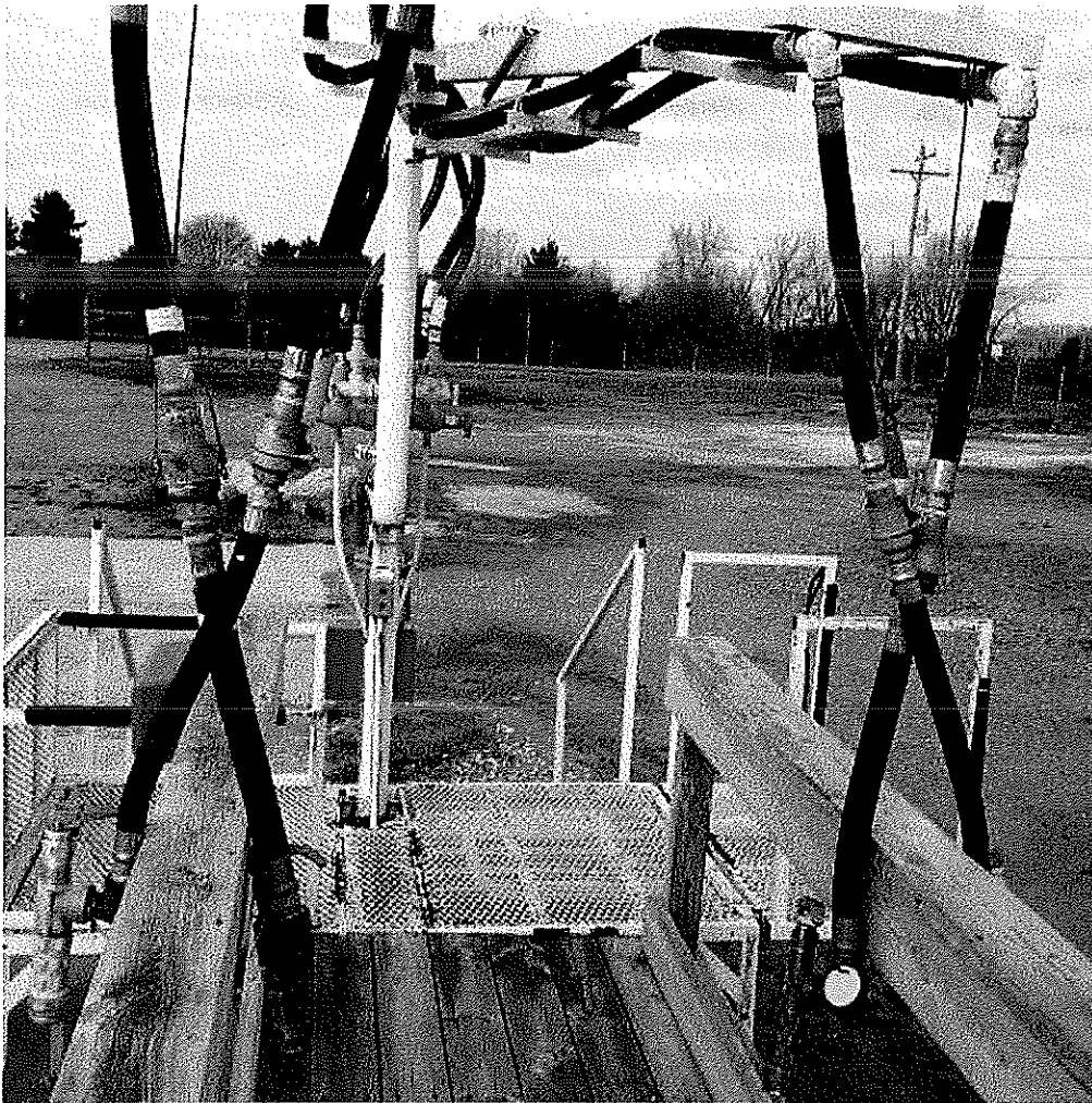
Image 6(013) : Nurse tank load out piping and break away valves
