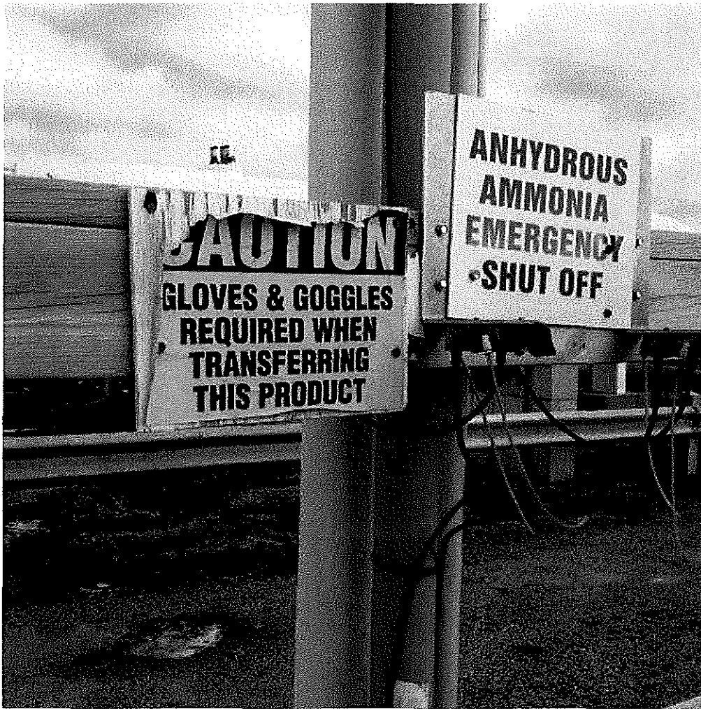
Image 5(011) : Emergency shut off valve at nurse tank loading
