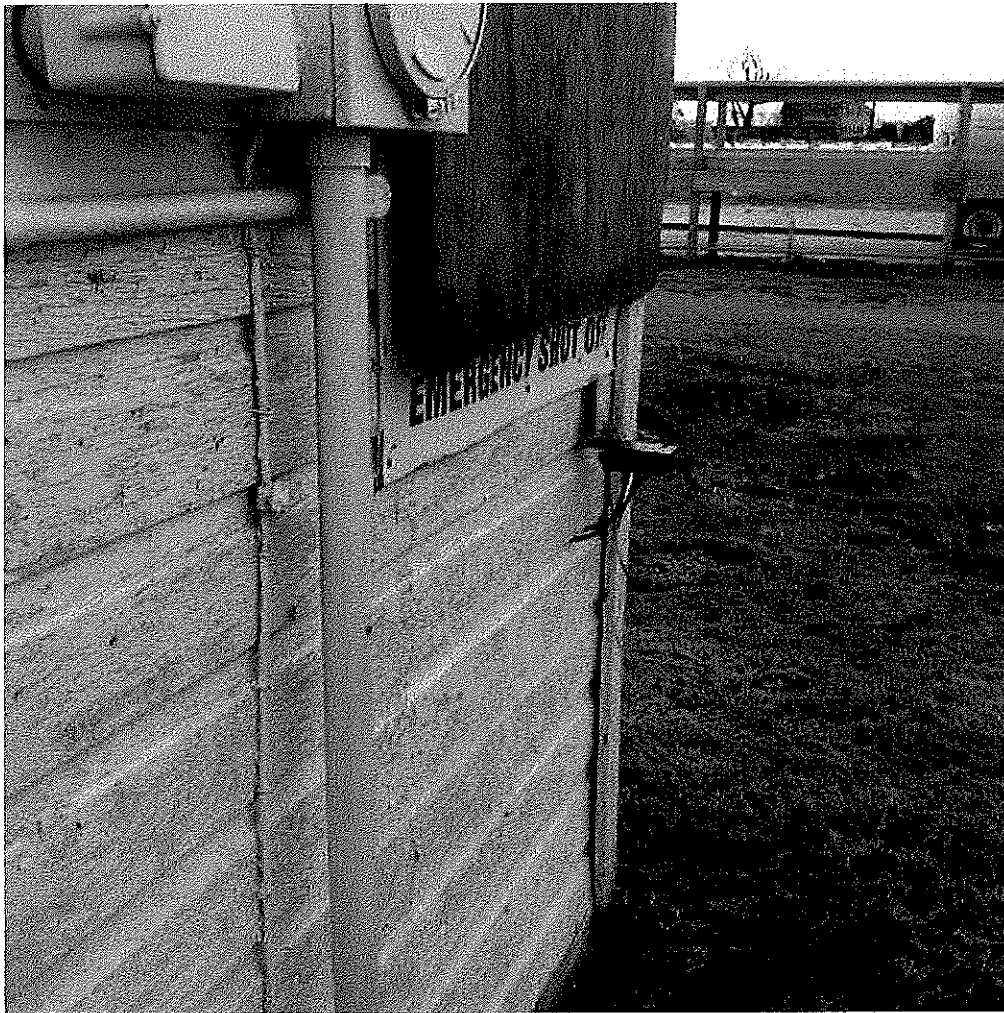
Image 3(007) : Emergency shut off valve
