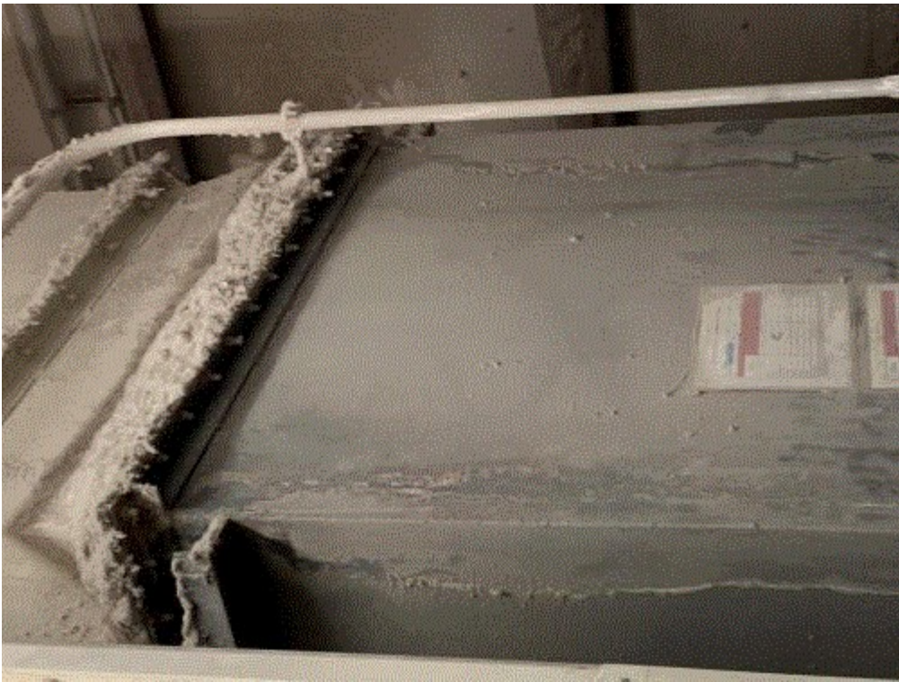
Image 2(Pneumafill Baghouse) : Dust/debris accumulating on the baghouse ductwork.
