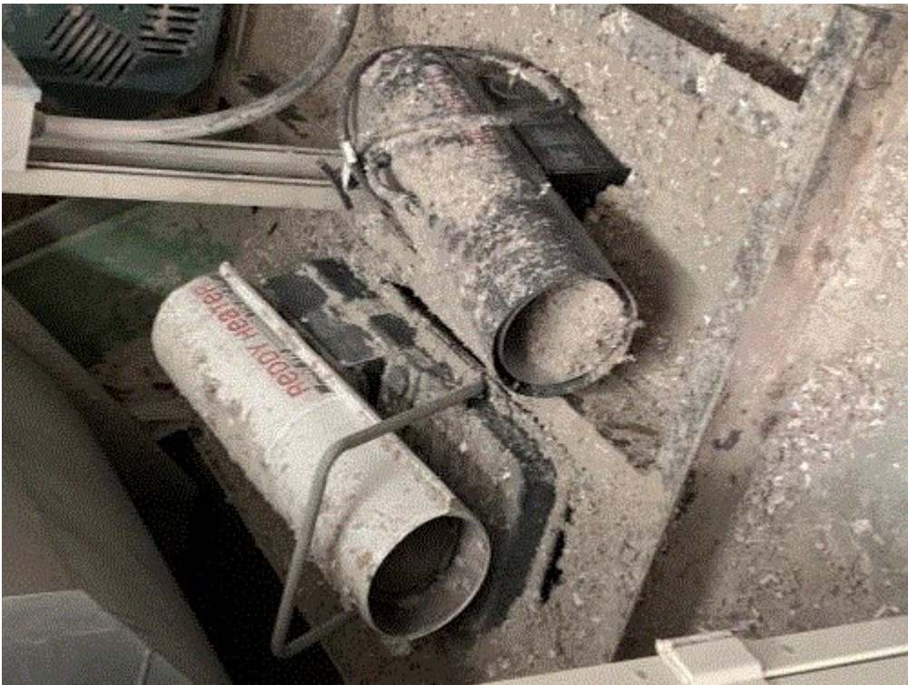
Image 3(Pneumafill Baghouse) : Dust/debris accumulating on other equipment near this baghouse.
