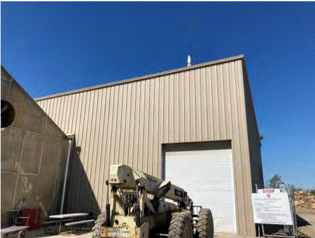
Image 3(003) : Boiler exhaust stack, with no opacity.
