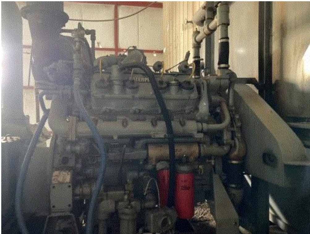
Image 2(Engine) : Caterpillar Engine at site
