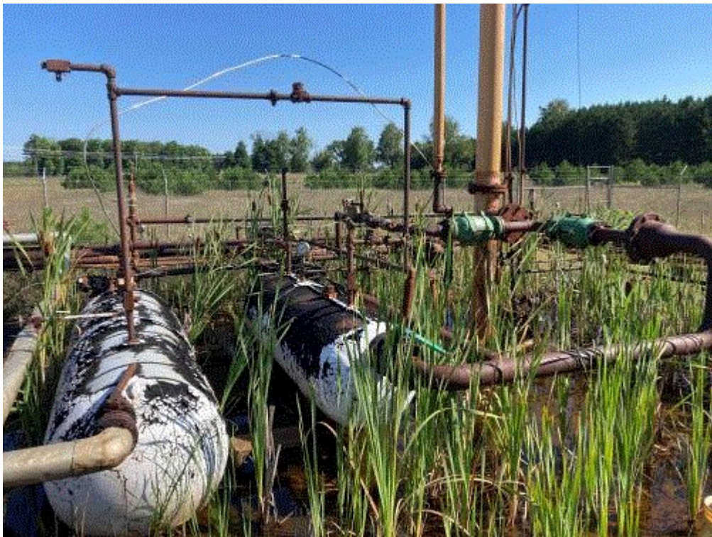
Image 4(Vegetation) : Overgrown Vegetation in flare secondary containment
