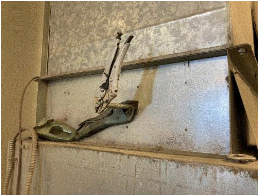
Image 2(IMG_0214.JPG) : May 14, 2021, Image of a broken damper actuator on the west plenum of the double-wide spray booth that has been replaced with vice grip pliers. This is one of two actuators on the double-wide spray booth that automatically adjust the pressure drop.
