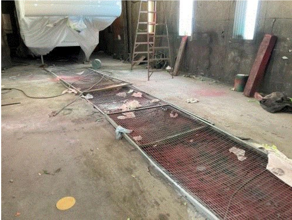
Image 1(IMG_0164.JPG) : March 17, 2021. East half of double-wide spray booth showing temporary grates while original grates are being cleaned in a burn-off oven at another facility.
