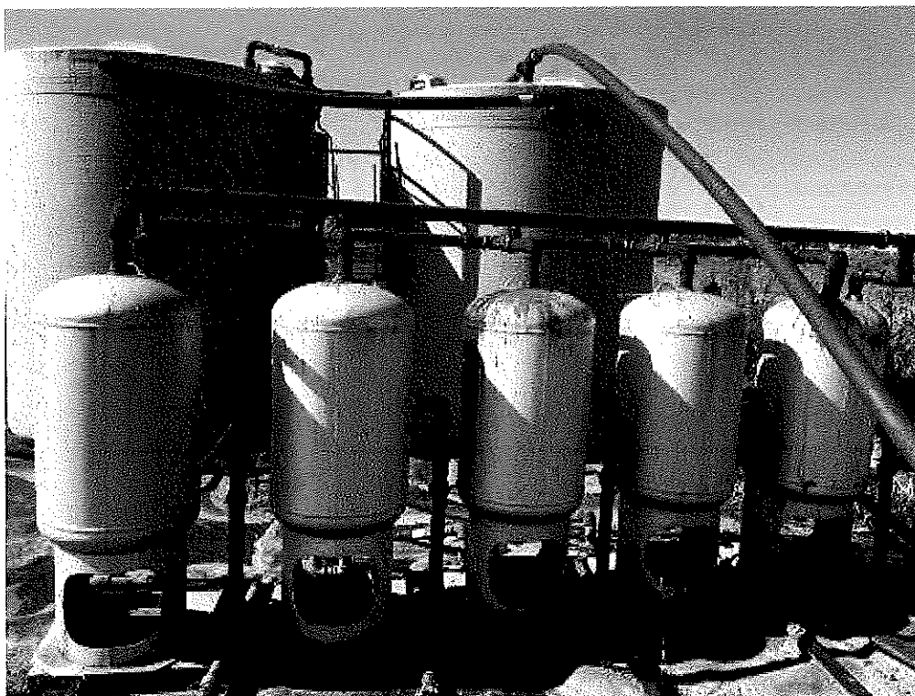
Image 2(Photo 2.) ; Photo 2. Reference photo of separator tanks and storage tanks. Perspective facing west.
