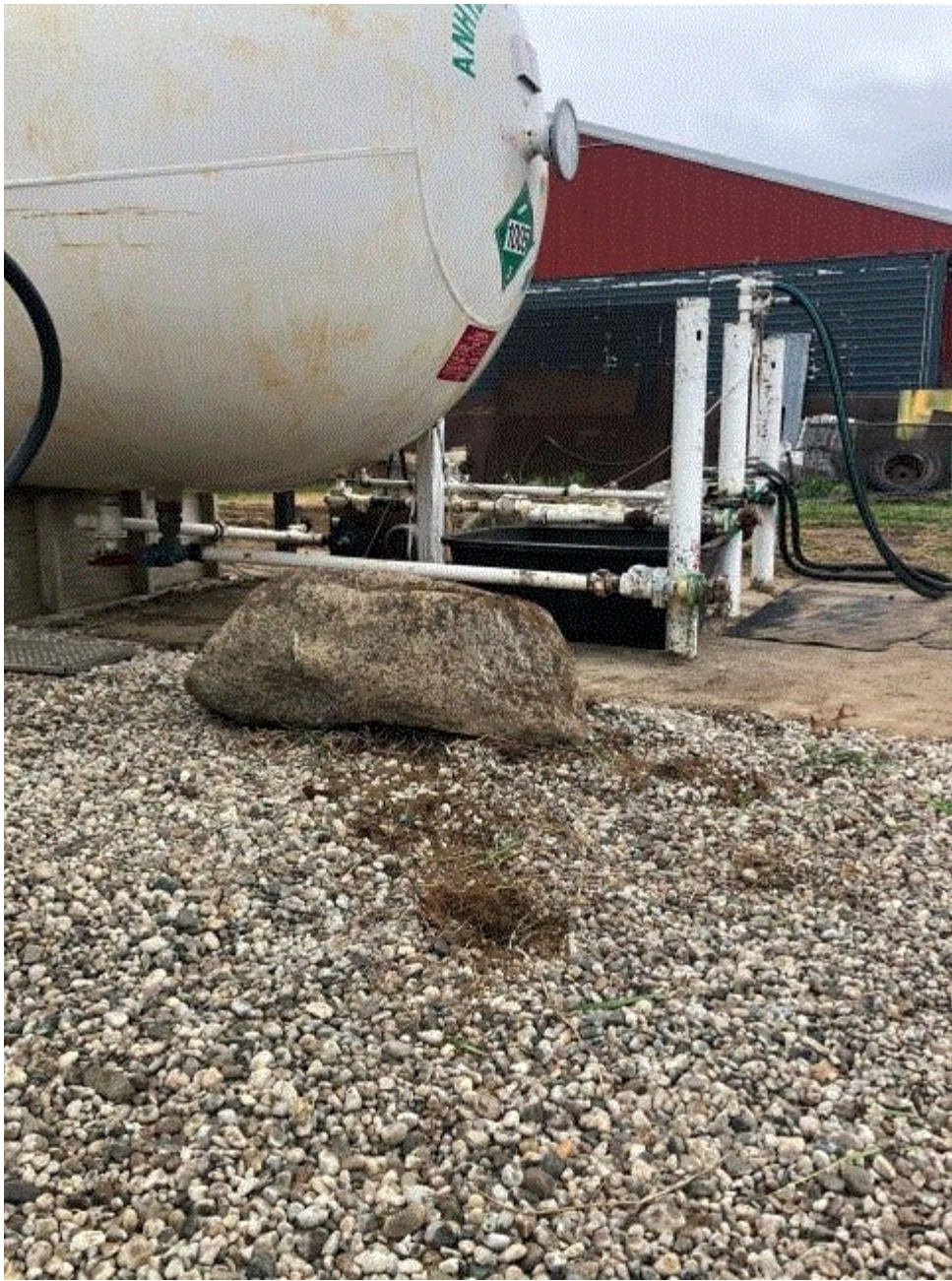
Image 1(Barrier 1) : Barrier installed on north side to protect pipes from accidental damage. Photo Credit: Travis Pidd
