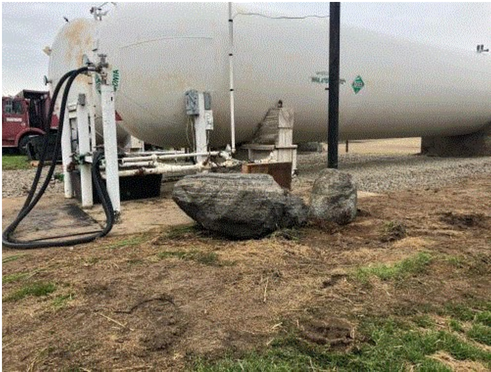
Image 2(Barriers 2) : South side barriers to protect anhydrous ammonia piping from accidental impact. Photo Credit: Travis Pidd
