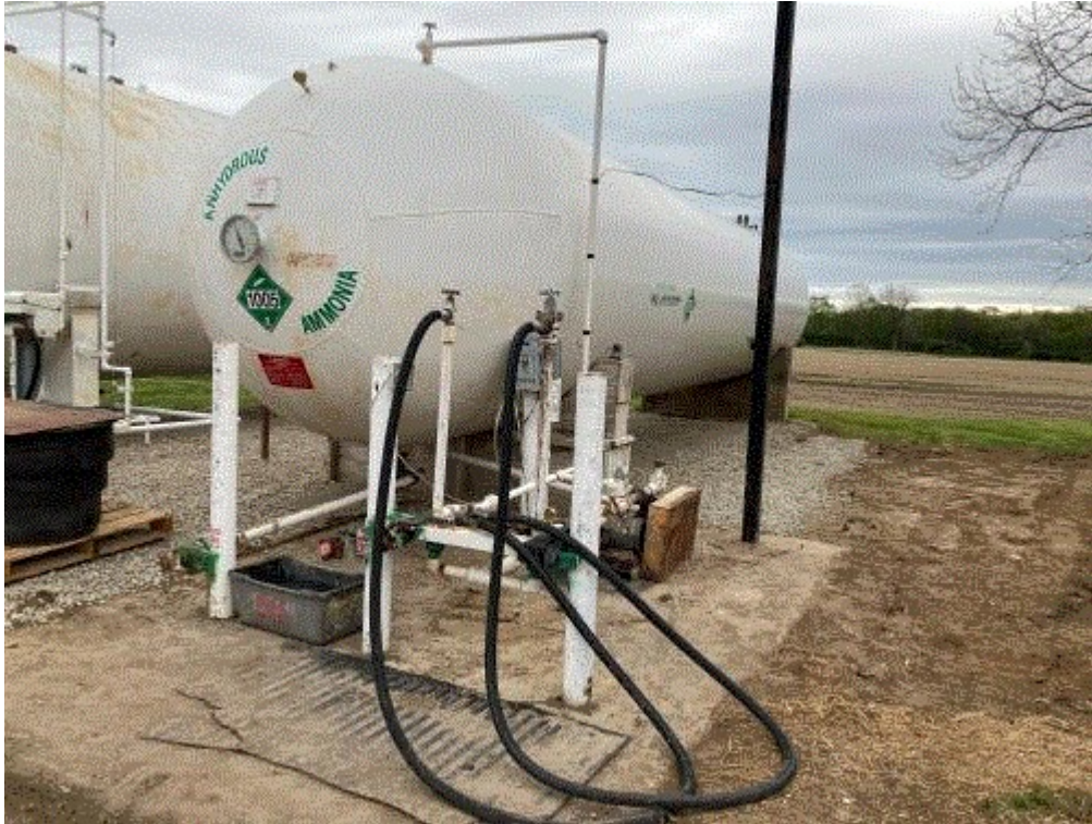
Image 6(Tank - full view) : Full view of the permanent storage anhydrous ammonia tank. Area to the right of the tank is where an unpermitted anhydrous ammonia tank (cited for Violation in 2016) has since been removed.
