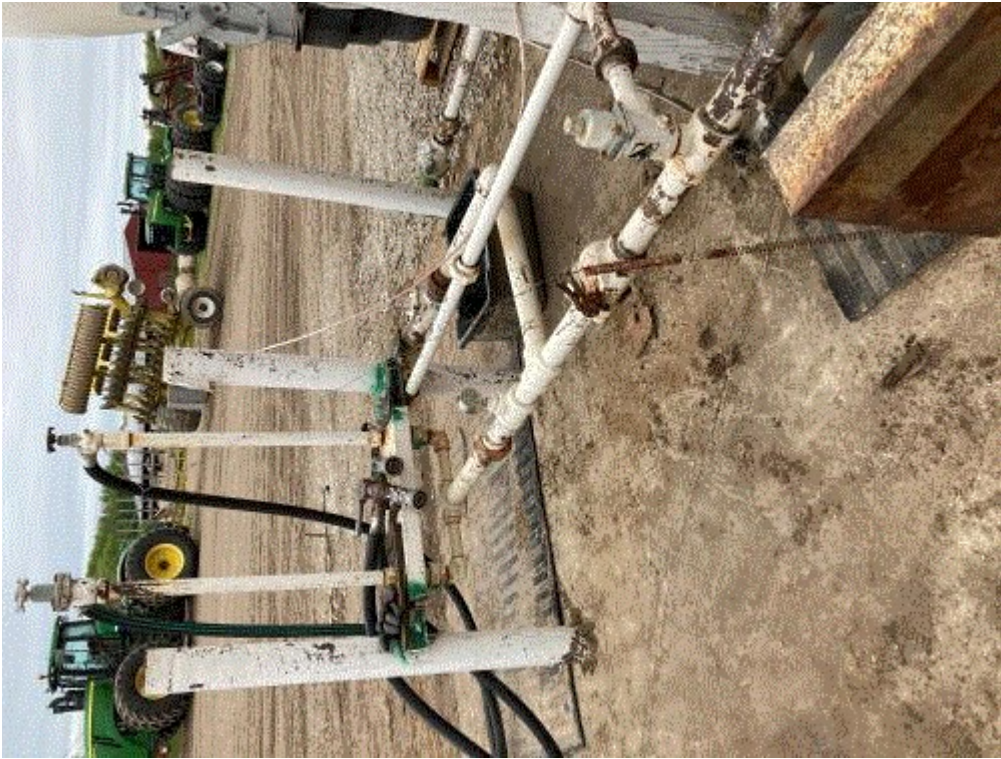
Image 8(Emergency shut off) : Remotely operated emergency shut-off system. Note: wire T's at the two lines on the bulk head, runs back to a spring system which is hooked to a lever-action valve.
