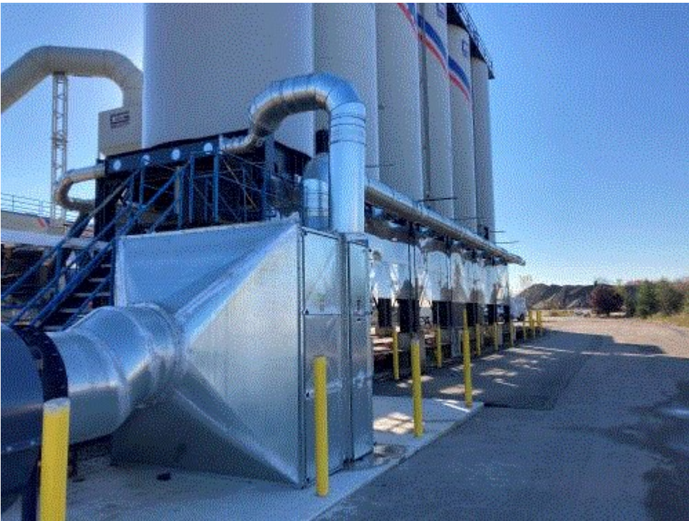
Image 3(Media filtration box) : Load-out control media filtration box.
