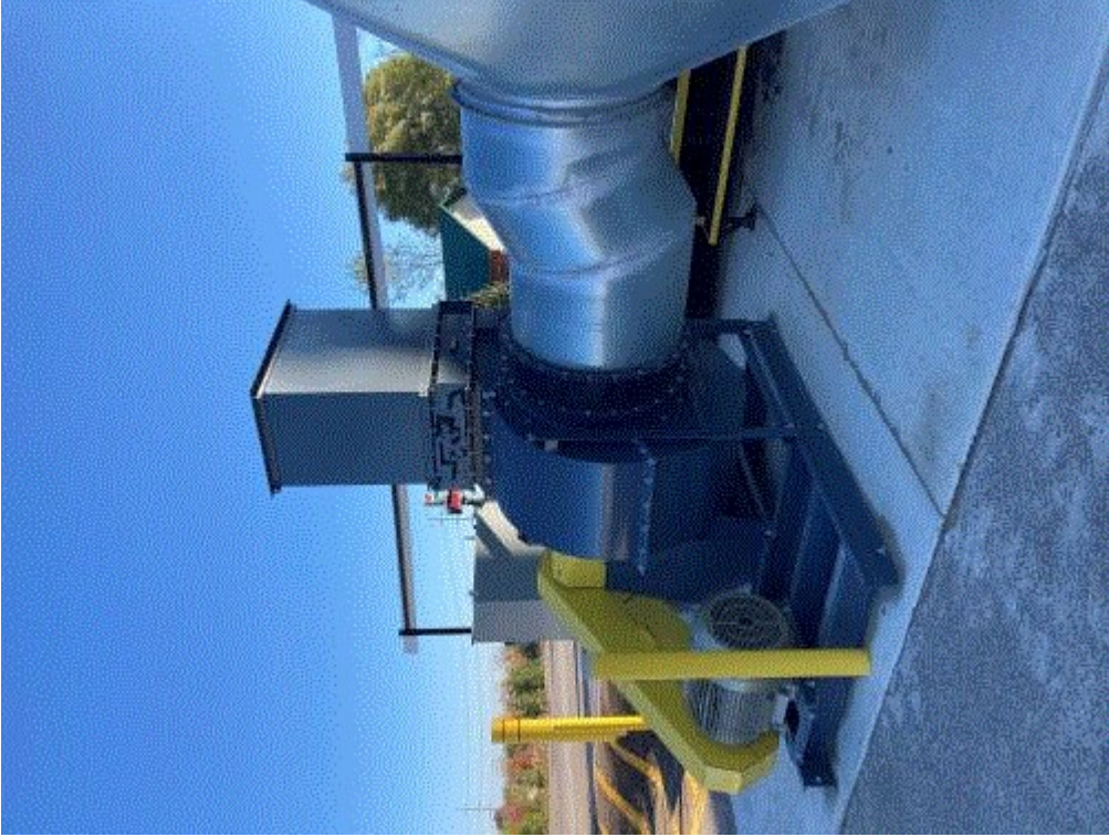
Image 4(Load-out stack) : Load-out media filtration stack.
