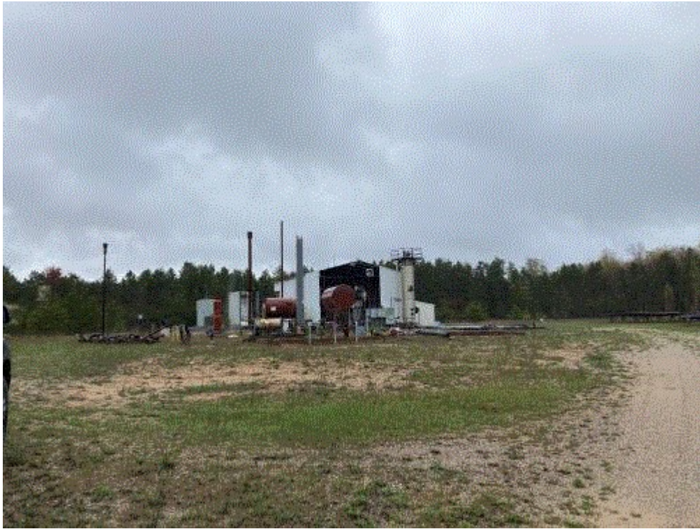
Image 1(Inspection Pics) : Overview of current equipment onsite
