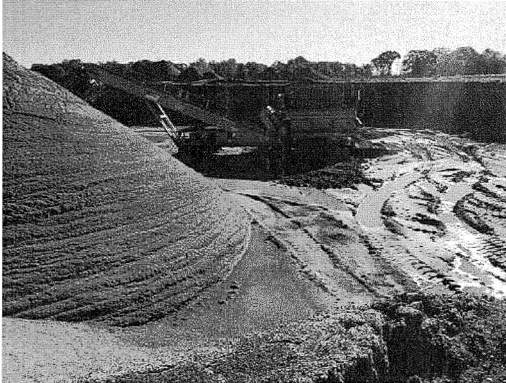
Image 14(Dry Screening) : Dry screening operation not accessible due to mud. This operation also has a diesel engine.
