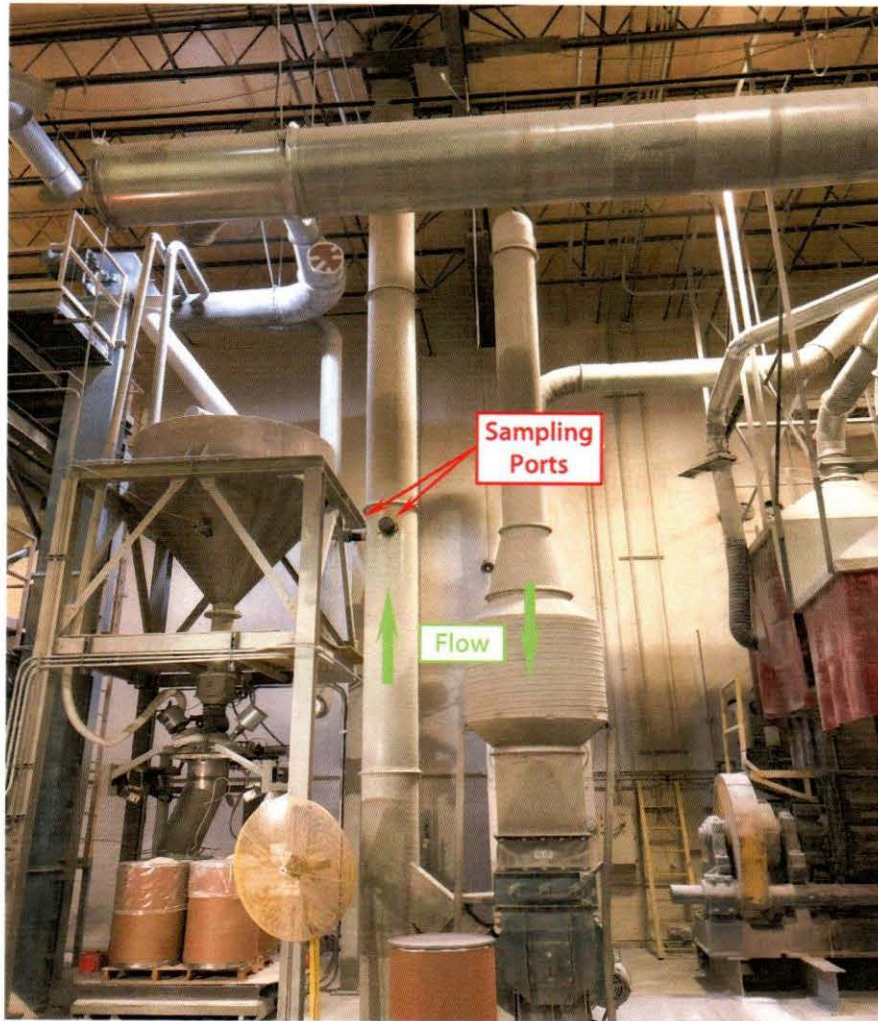
Figure 2-4. Liquid Bay Sampling Location
