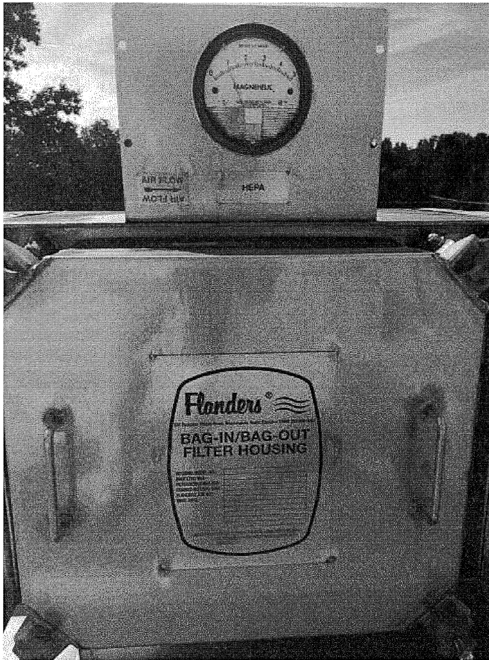
Image 3(HEPA Manometer 2) : EUSNAP manometer reading from BeO HEPA filter. ~1 in. H2O
