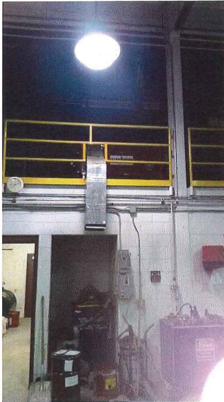
Image 2(CE3) : Location of CB-2500 furnace on mezzanine in maintenance garage
