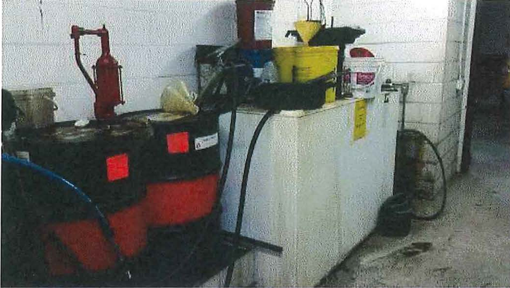
Image 1(CE2) : Waste-oil tank and drums
