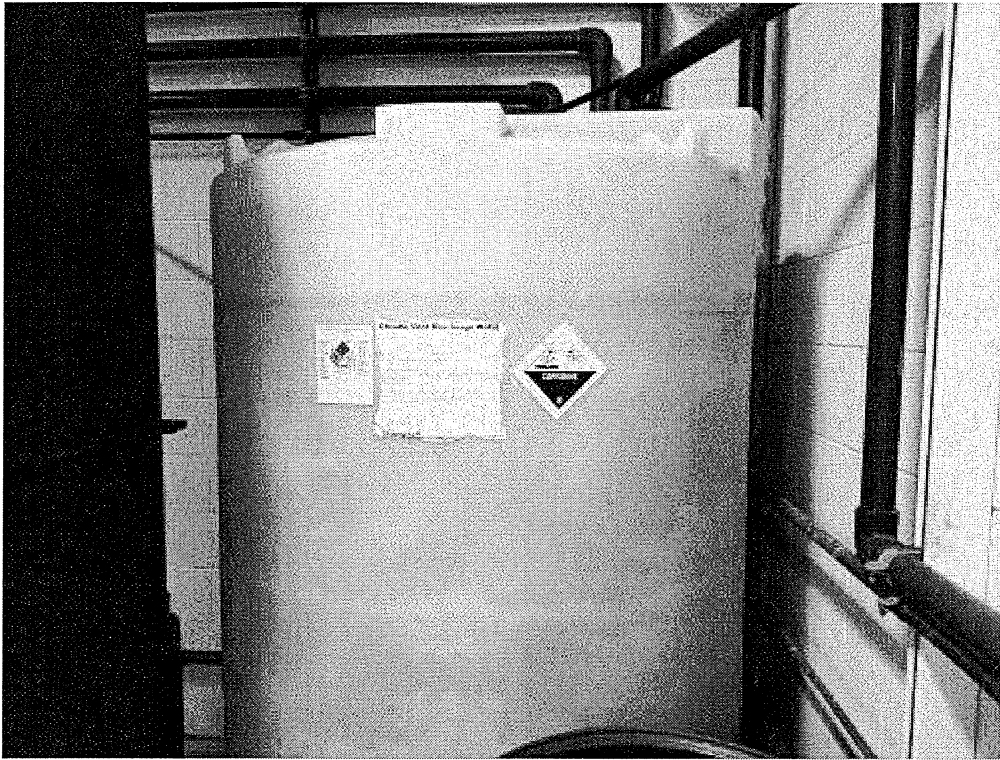
Image 6(Chromium Waste) : Wastewater tank from Chromium scrubber (SC1)
