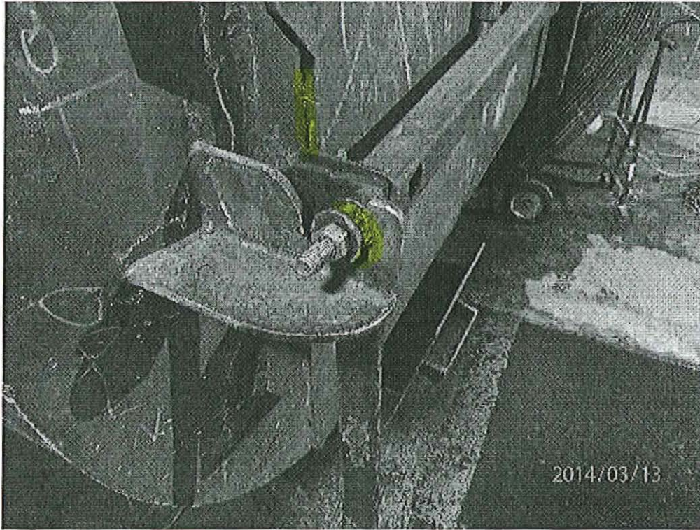
Image 4(IAR Combustion Unit) : Combustion unit door weld
