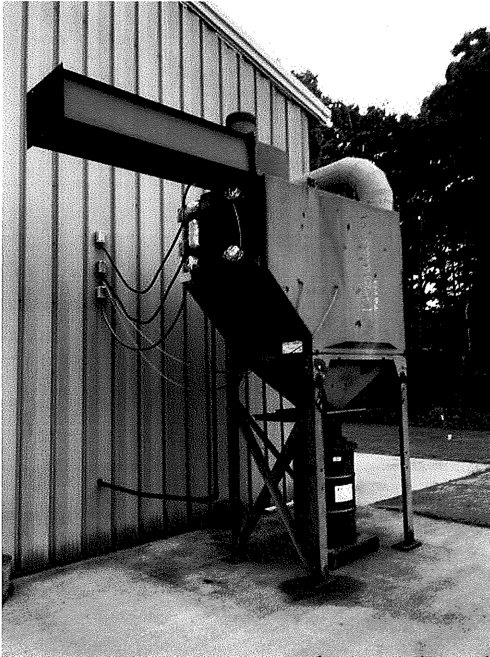
Image 1(Catridge filter) : one of the cartridge filter baghouses for 2 of the shot blasting wheelabrators
