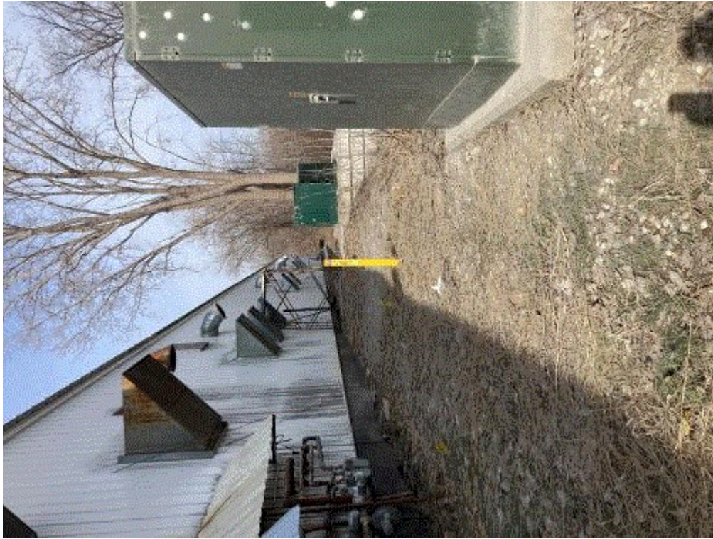
Image 3(Baghouse exhausts) : Baghouse exhausts and air intakes for paper processing and pelletizing lines.
