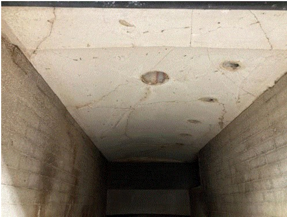
Image 3(IMG 0402) : Upward view of the front of EUCREMATORY1 primary combustion chamber ceiling. No significant cracks were observed. Cremains are swept to the rear floor of the primary combustion chamber. The cremains are then collected through a rear door.
