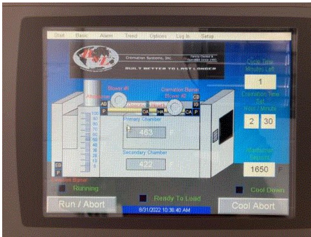
Image 8(IMG_0395) : EUCREMATORY1 control panel. Note that the Afterburner (secondary combustion chamber) Setpoint is 1650F, which appears to support Kenneth Allen Sr.'s assertion that the low-temperature records are due to a chart recorder calibration error.
