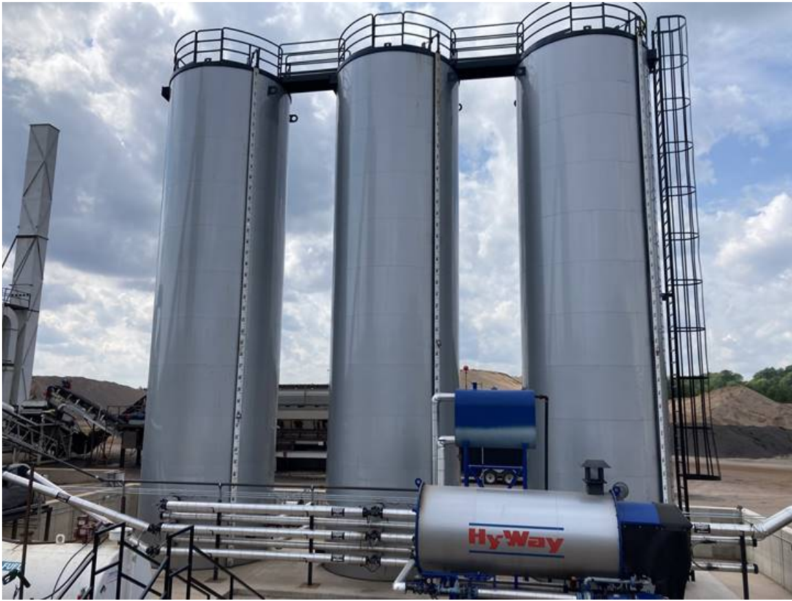
Image 1: Three AC tanks
