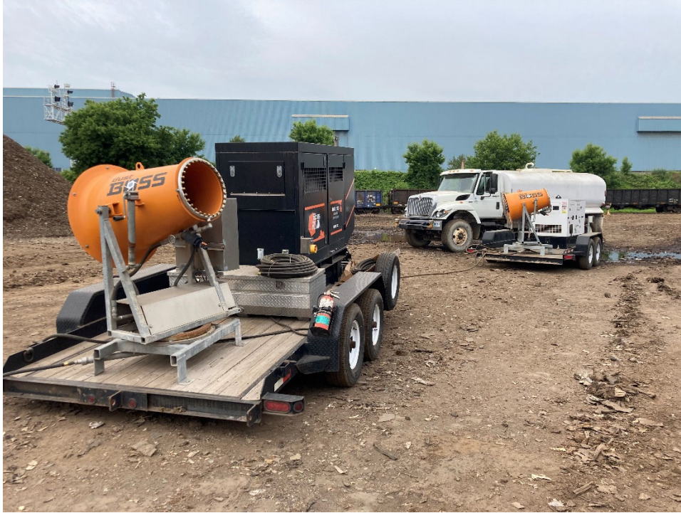
Photo of Dust Boss and water truck used to mitigate fugitive dust
