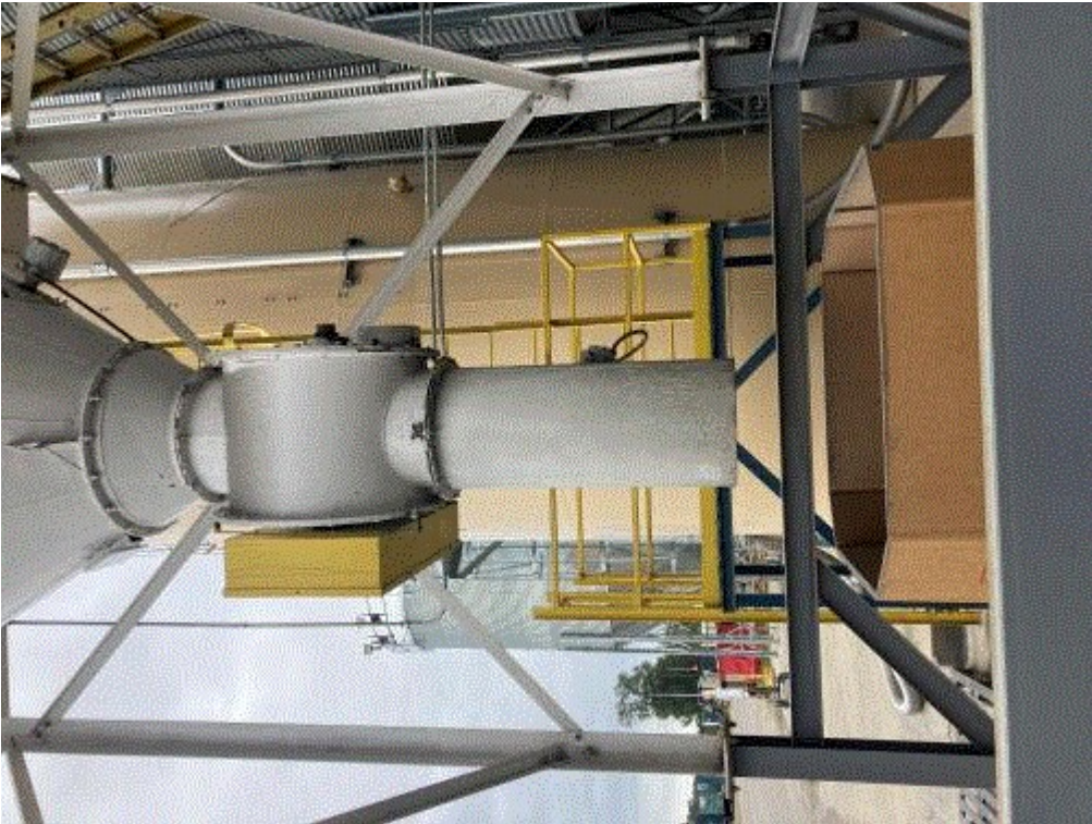
Image 2(Shredder 2) : Shredder 2 baghouse discharge. View photo one turn clockwise.
