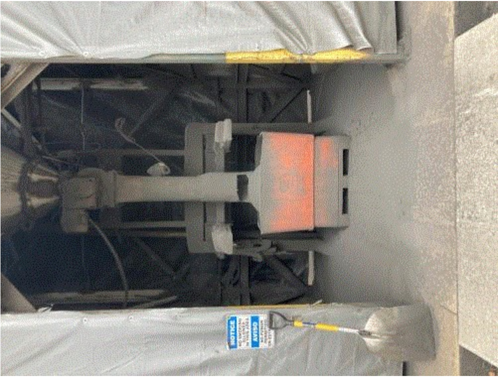
Image 1(Shredder 1) : Shredder 1 baghouse discharge. View photo one turn clockwise.
