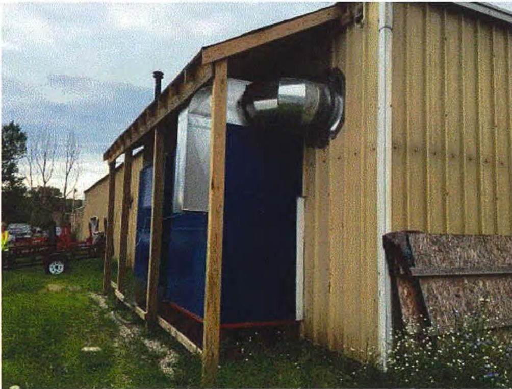
Image 1(3) : Dust collectors on the sand blasting process.
