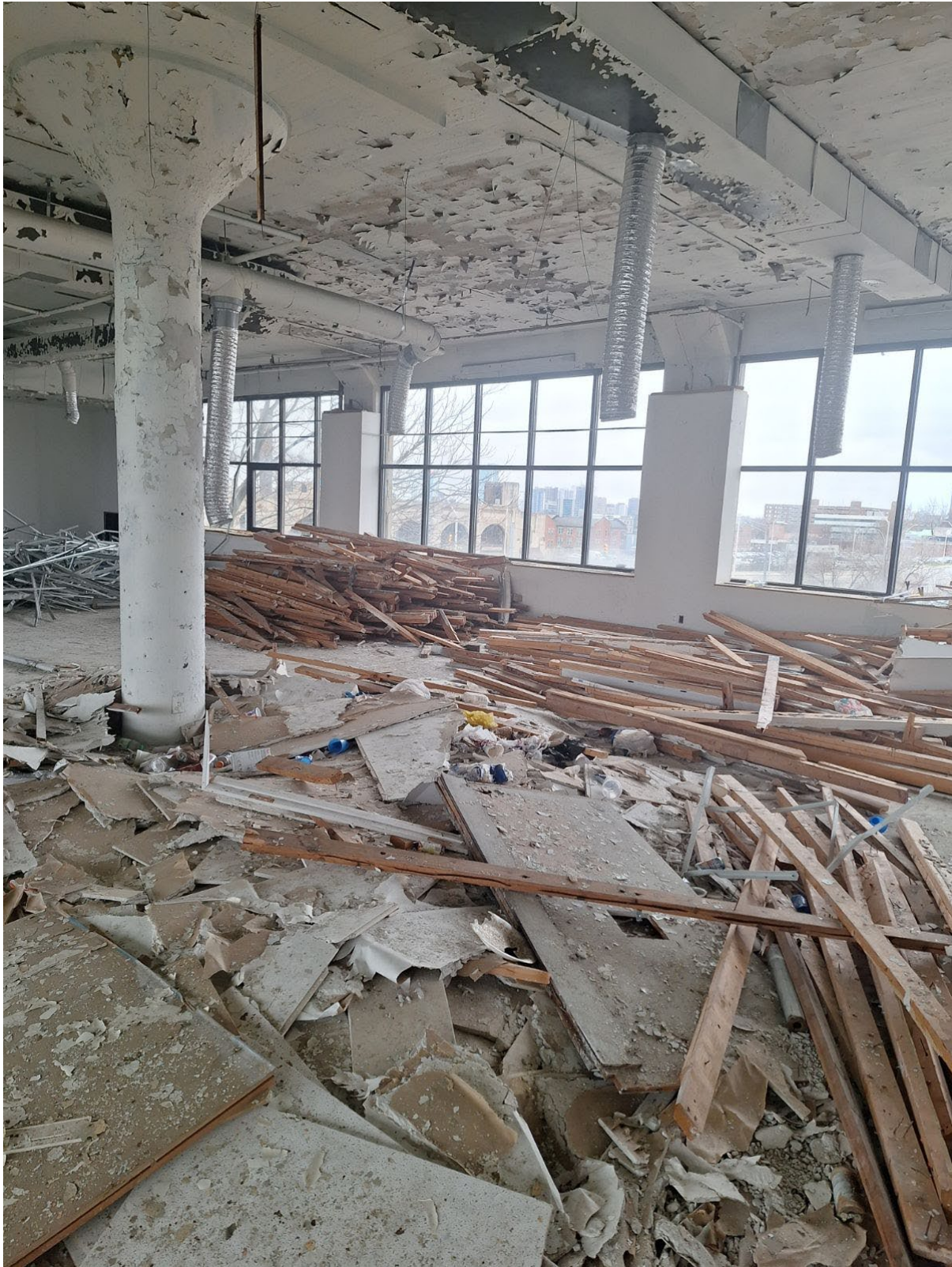
Photo 1: Photo taken November 20, 2023 of 1953-1959 E Jefferson interior at fourth floor taken by Poe Restoration employee prior to beginning our debris removal work. This gutting/demo was done prior to our arrival.
