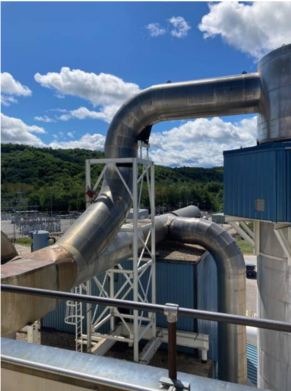
Image (1): Exhaust system and SDA tower
