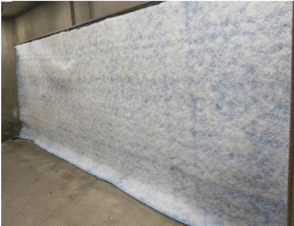
Image 2(image000000(4).jpg) : RESOLUTION OF COMPLIANCE CONCERN: April 12, 2022, Image of new dry filter media and installation, which appears to correct the AQD's concerns about the potential of exhaust
