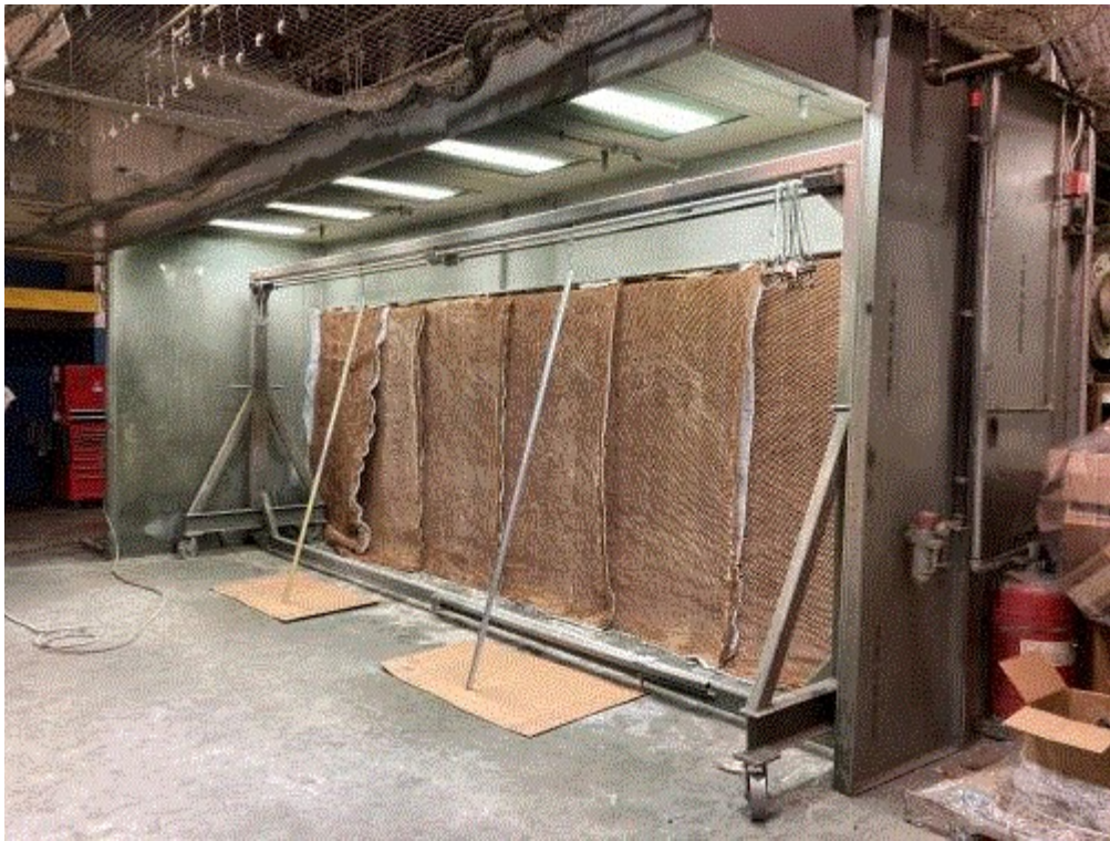
Image 1(IMG_0299.JPG) : Former chain-on-edge spray booth. Note the gap in the overlapping exhaust filters on the left. The gap presents a potential bypass path.
